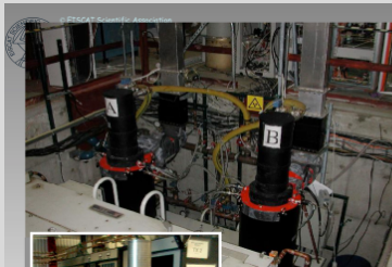
Two 1-MW UHF klystrons (930 MHz) at Tromsø.
