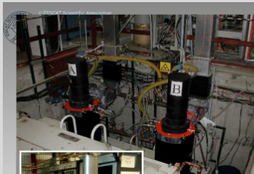
Two 1-MW UHF klystrons (930 MHz) at Tromsø.
