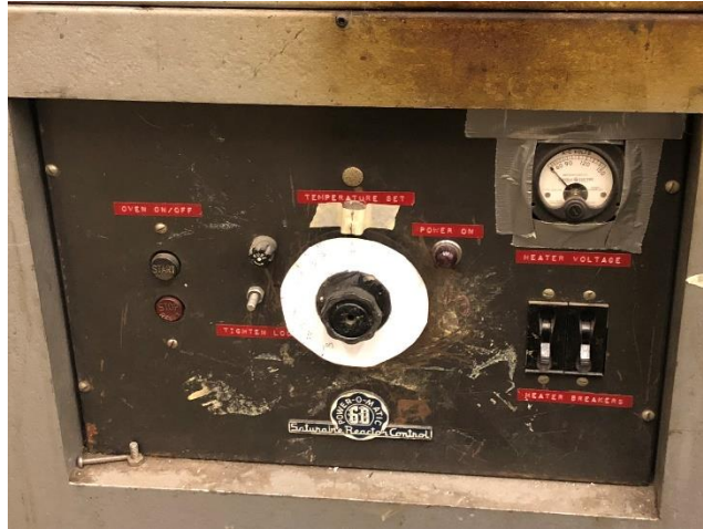
^Control panel with START/STOP buttons, dial, and heat breakers
