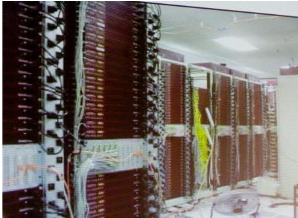
Google Data Center (current capacity hard drives >2Tb)
